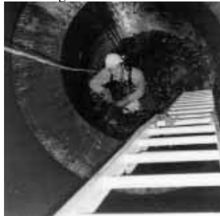
Photograph 5.7 Manually cleaning the CDS unit
